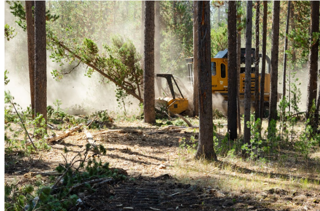
A masticator thins and mulches trees to reduce the fuel load in a forest outside Yellowstone National Park. By creating defensible space this project helps protect nearly 2,000 structures adjacent to the park from fire. (NPS/Jacob W. Frank)
